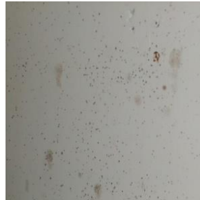
Water leaks = mold hazards
