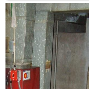
Broken ducts = higher heating bills
